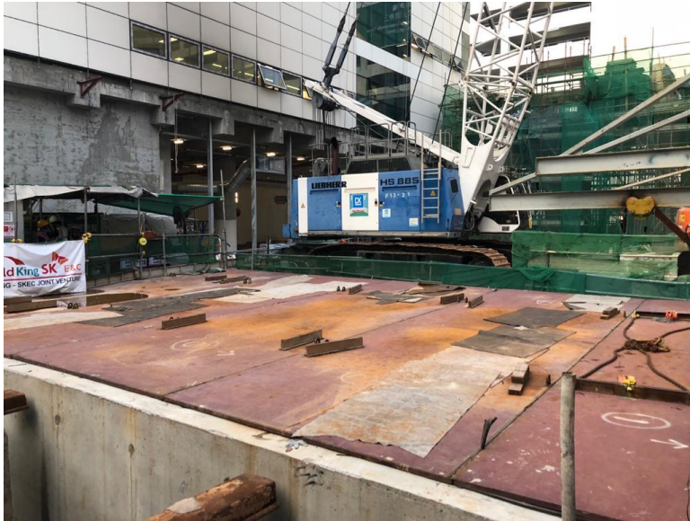
Figure B3: Closure of Acoustic Panel
