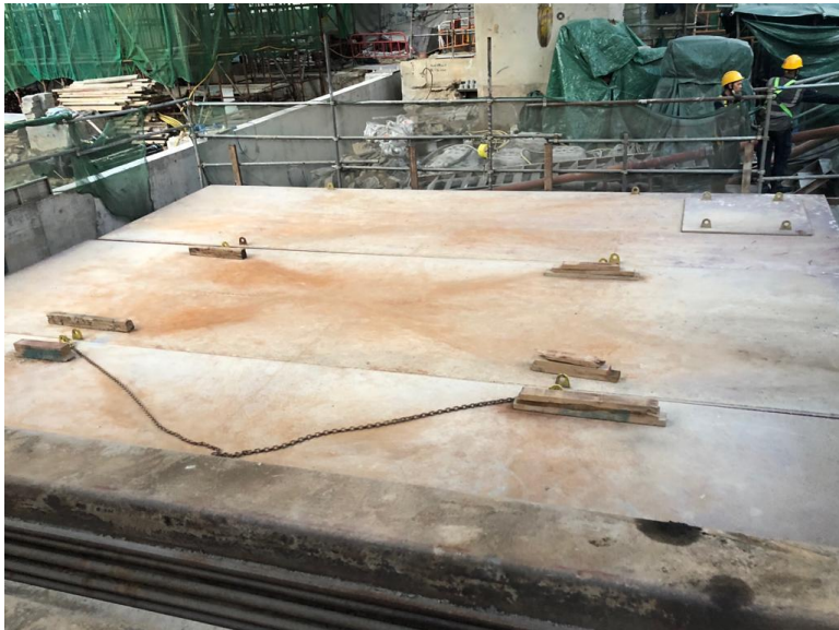
Figure B4: Closure of Acoustic Panel
